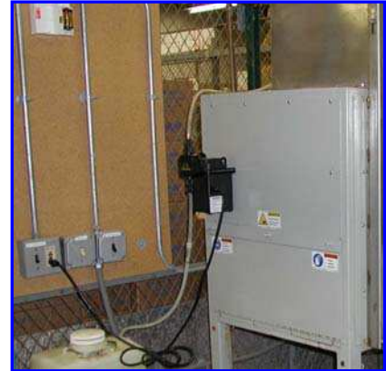
Typical Metering Pump Install
